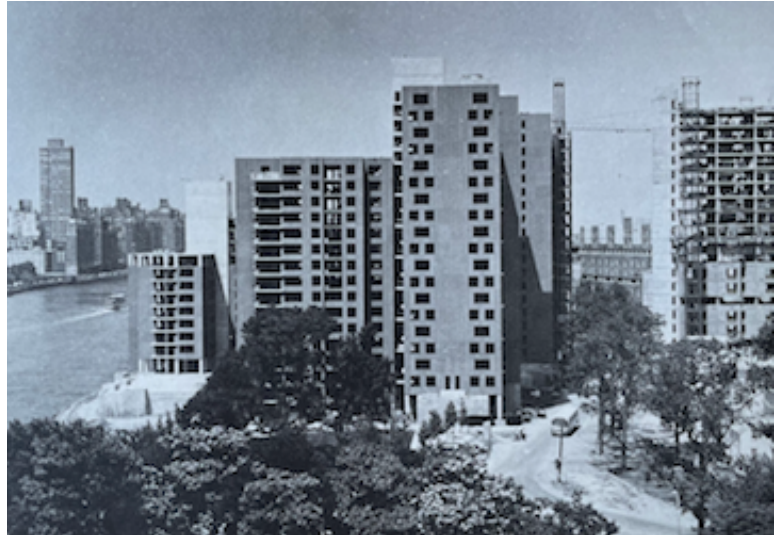
View north along Main Street of Rivercross apartment building under construction. From Roosevelt Island Development Corporation promotional brochure, 1974.
